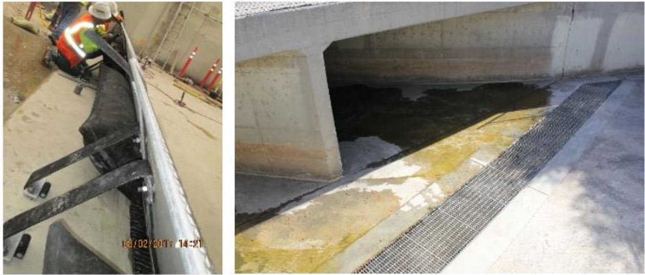
Figure 5 Inflatable Rubber Dam (Left) and Grated Drop Inlet (Right)
