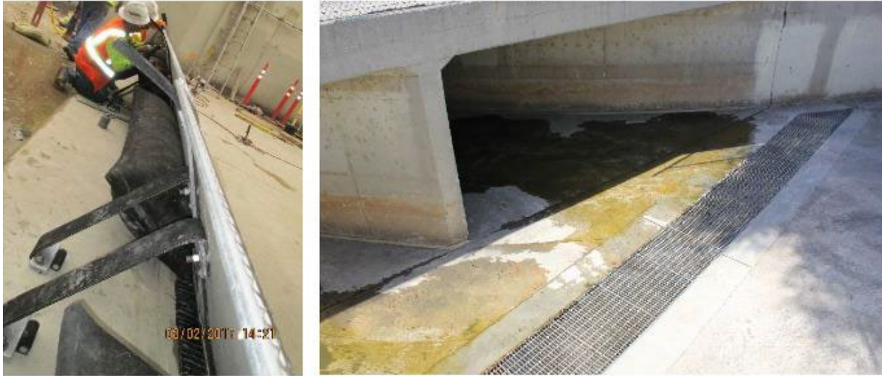
Figure 12 Inflatable Rubber Dam (left) and Grated Drop Inlet (Right)
